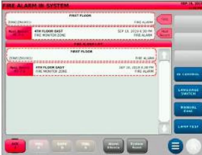
Figure 10: First and Most Recent Alarm Display
